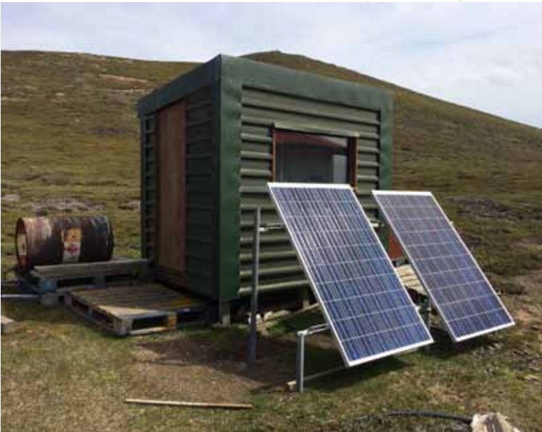
Saunders Island - Solar Panels and power storage shed
